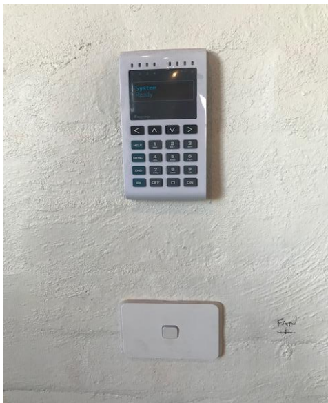
Boiler House can be disarmed/armed on this panel, or from the panels at the main theatre entrance, or office entrance
