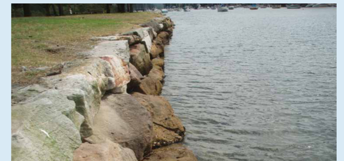
Seawall made from boulders of various size and shape with spaces between boulders providing sheltered habitat for wildlife (Source: Department of Environment and Climate Change NSW, 2009).
