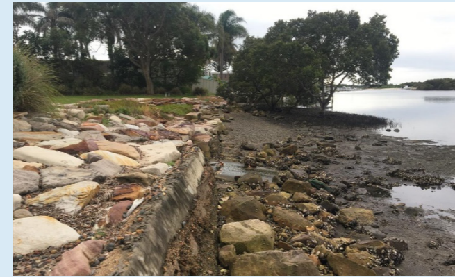
A rock revetment used to stabilise an eroding foreshore in an area that experiences ocean tides. The treatment retains and encourages foreshore vegetation (mangroves). It uses loose rock walls to protect against erosion and provide habitat, creates tidal pools for saltmarsh, the revetment has a sloping bank at high water mark to catch sea grass wrack, and steps down to provide access to the water.
