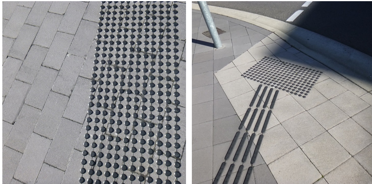
Example of bladed-shaft Hazard warning and directional warning systems installed at Charlestown Town Centre.
