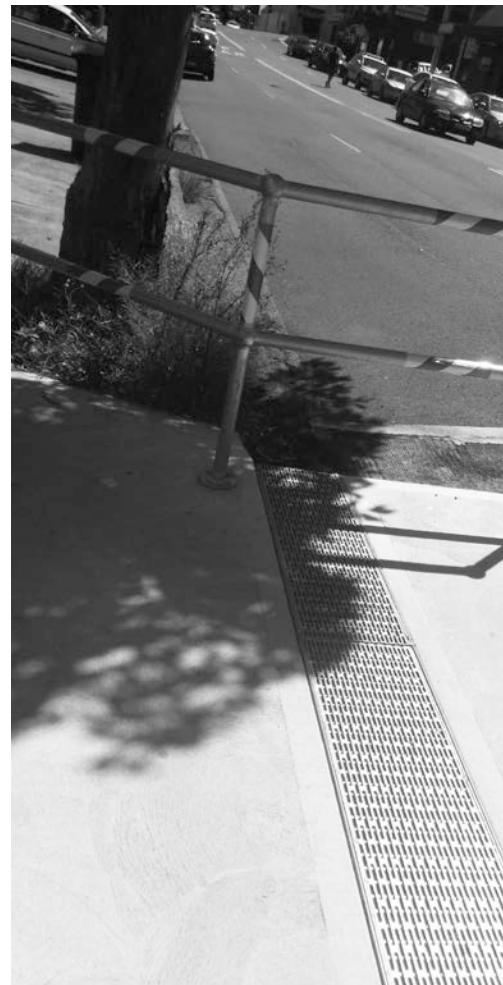
Existing drainage grate on kerb extension, Harrison St Cardiff
