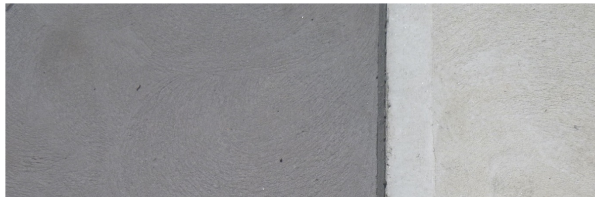
Existing dark grey coloured concrete next to standard concrete, Main Rd, Cardiff.
