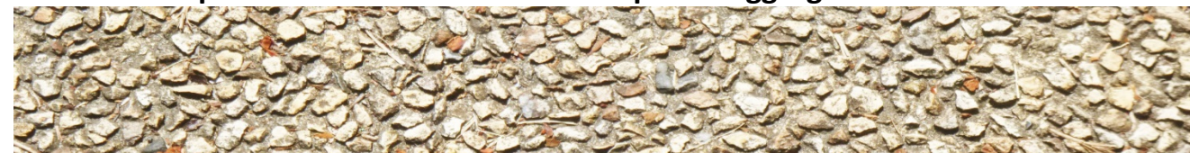
Example of existing coloured concrete with exposed aggregates at Belmont Town Centre
