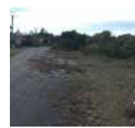
Blacksmiths: Ungula Road debris following a flooding event
