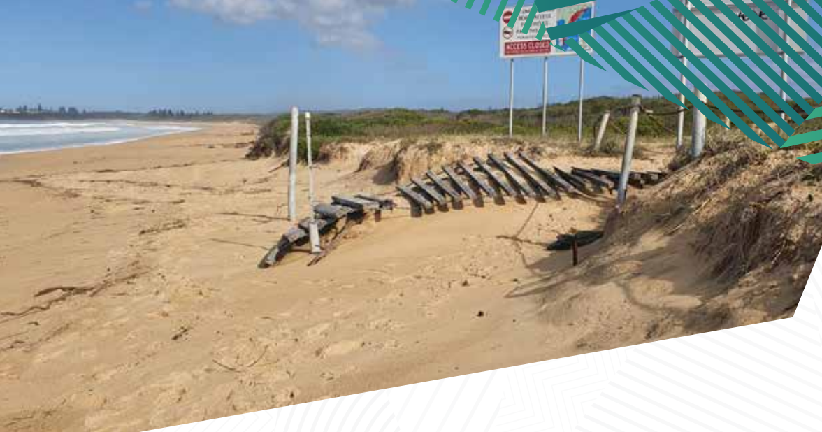
Erosion of beach and dune (including vegetation) Blacksmiths Beach near Awabakal Street, May 2021.
