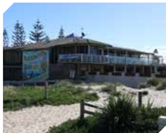
Over time Blacksmiths and Caves Beach Surf Clubs will be subject to coastal hazards and require replacement or relocation.
